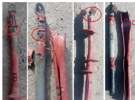
Fig. 3 Damaged cable terminations in case 2.
