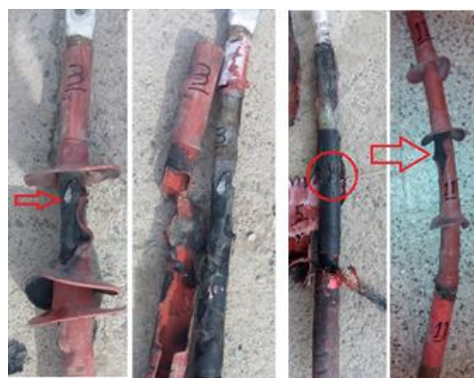
Fig. 2 Damaged cable terminations in case 1.
