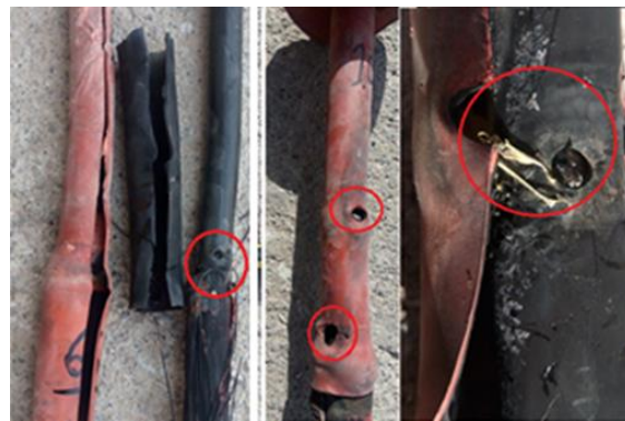
Fig. 1 Damaged and burned cable terminations in main triple point region.
