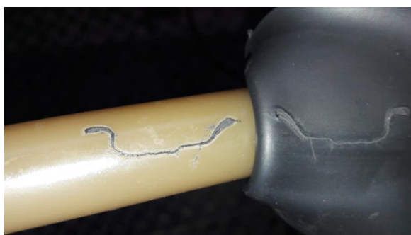
Fig. 11 Fault under SG because of wet and pollution.
