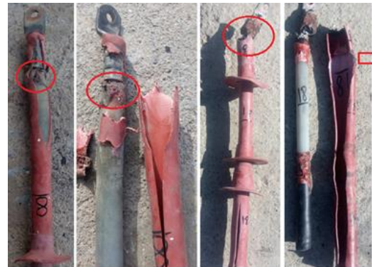
Fig. 3 Damaged cable terminations in case 2.
