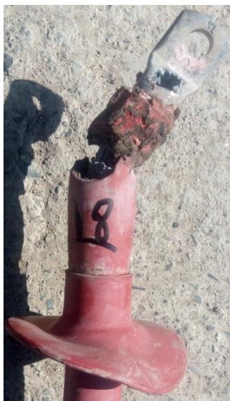
Fig. 16 Damaged cable termination because of breakdown and electro-mechanical forces.
