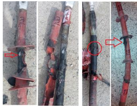
Fig. 2 Damaged cable terminations in case 1.
