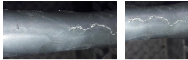
Fig. 10 Treeing effect in the area with void under SG.
