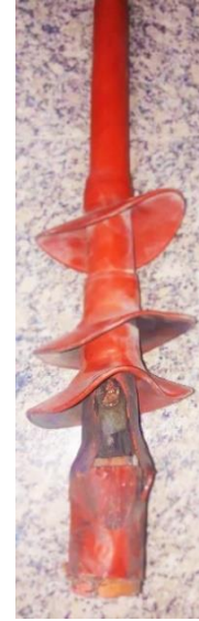
Fig. 11 Punctured cable termination in triple point area (Case 1).
